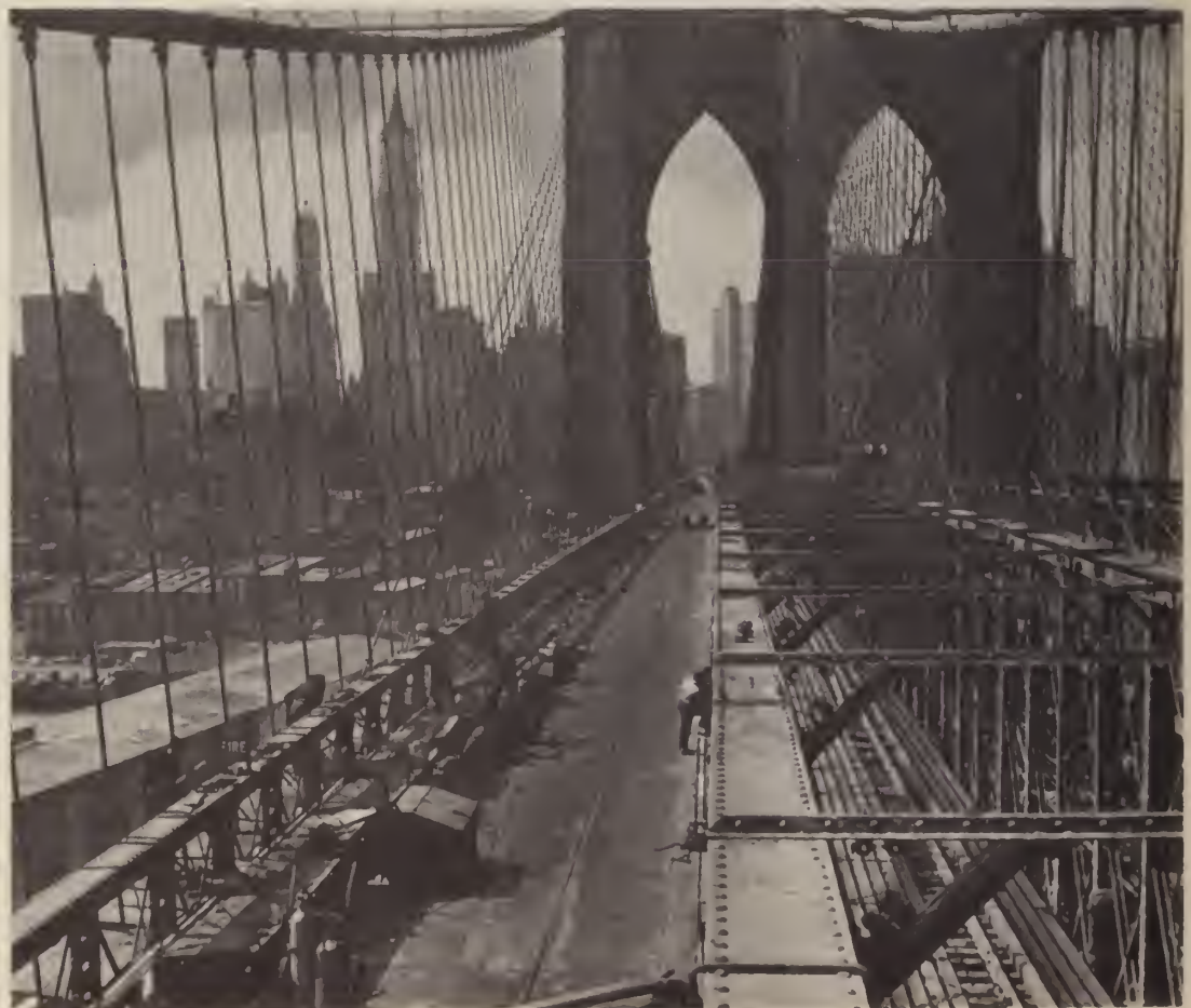
Holes are drilled in the old top chords of truss prior to raising height of truss at outer edge of Bridge.
